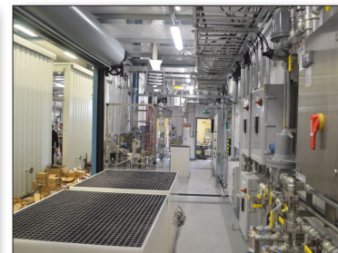
Tote slips with containment
