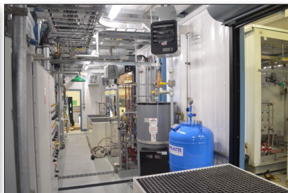
Environmental and safety systems
