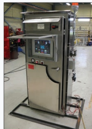
PLC with touch screen HMI
